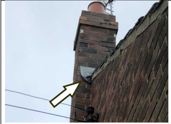
Photo 7: PRF – Gap under Chimney lead flashing
