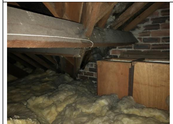
Photo 15: PRF - Large area of torn bitumen felt underlay
