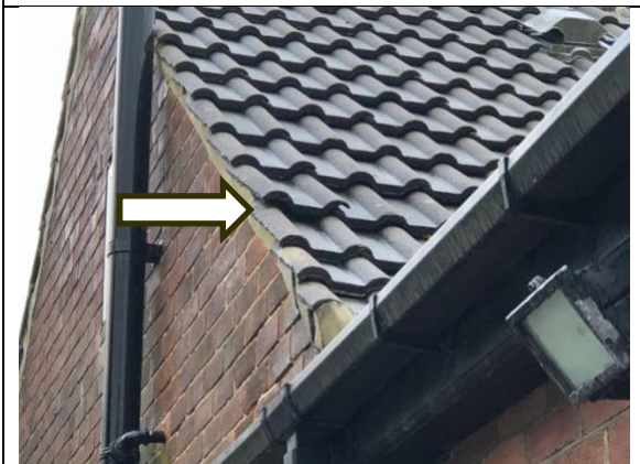
Photo 9: PRF – Gap under raised tile
