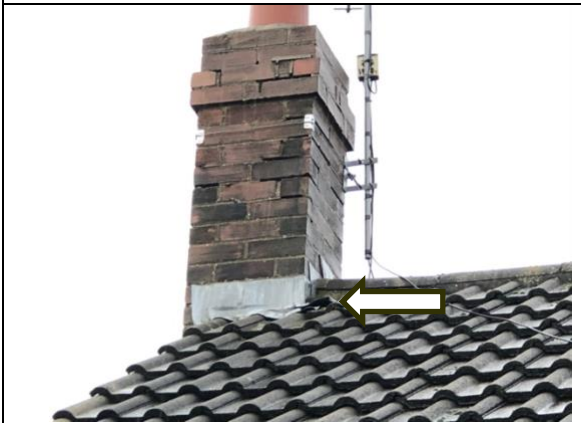
Photo 8: PRF – gap under Chimney lead flashing
