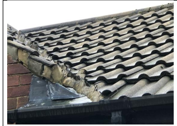
Photo 10: PRF – gaps in mortar and missing mortar along roof valley on southwest aspect
