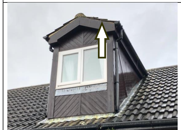
Photo 6: Dormer window on rear aspect with PRF – missing mortar.
