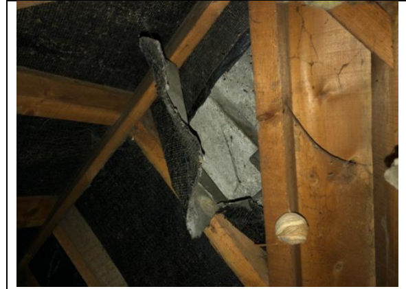
Photo 14: PRF - Large area of torn bitumen felt underlay
